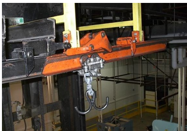
Orange lifting rail mates with black overhead monorail
